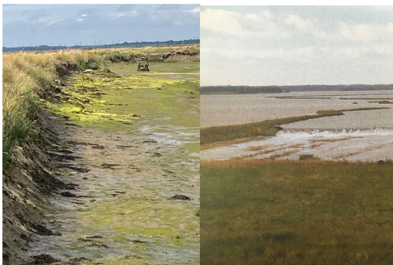
Photos : Wall being undermined from the rear north side and, right, inner wall at exceptional tide flooding with spur beyond which is being undermined from the rear as in detailed photo.
