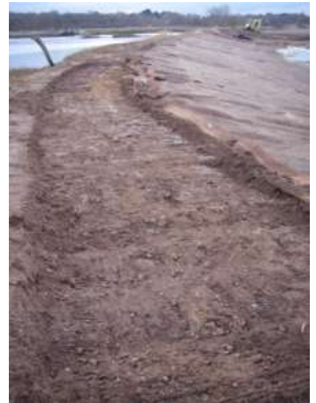
Excavation for crushed concrete foundation. This photo illustrates the curve of the path at this location (looking west)
