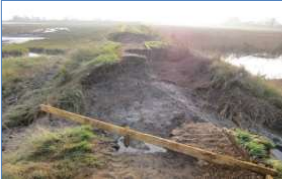
An example of an estuary defence footpath damaged in December 2013 surge
