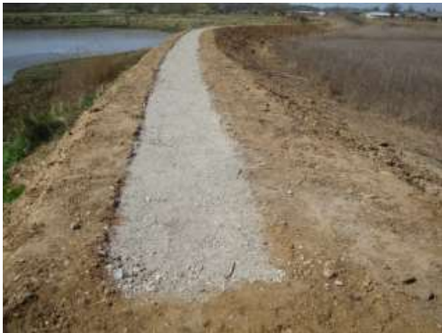
Crushed concrete, prior to compaction, on first section of the wall (looking east)
