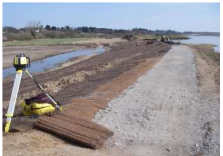
The only thing left to do is to seed the turf reinforced mesh. As well as a grass surface on the landward slope it is hoped that vegetation will re-establish itself along the path margins.
